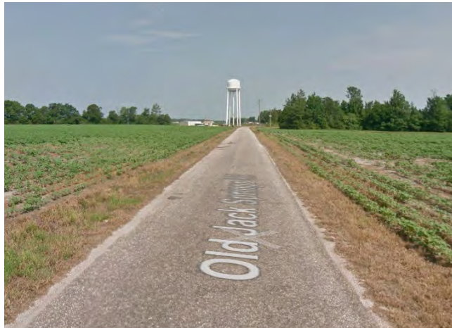
FLAT TERRAIN ALONG OLD JACK SPRINGS RD CONTRIBUTING TO POOR DRAINAGE
