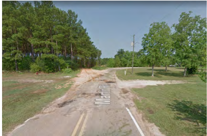
WORN SURFACE AT MARTIN RD/SMALL PINES RD
